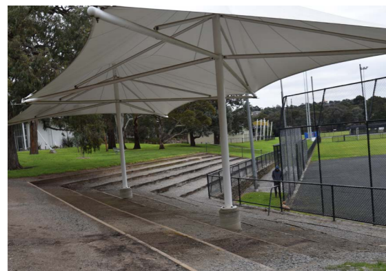
The existing softball spectator area, proposed to be refurbished as a part of this package.
