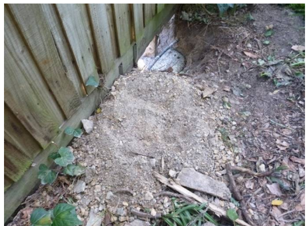
View of post hole excavation and associated spoil in the north of 35-37 Regent Street
