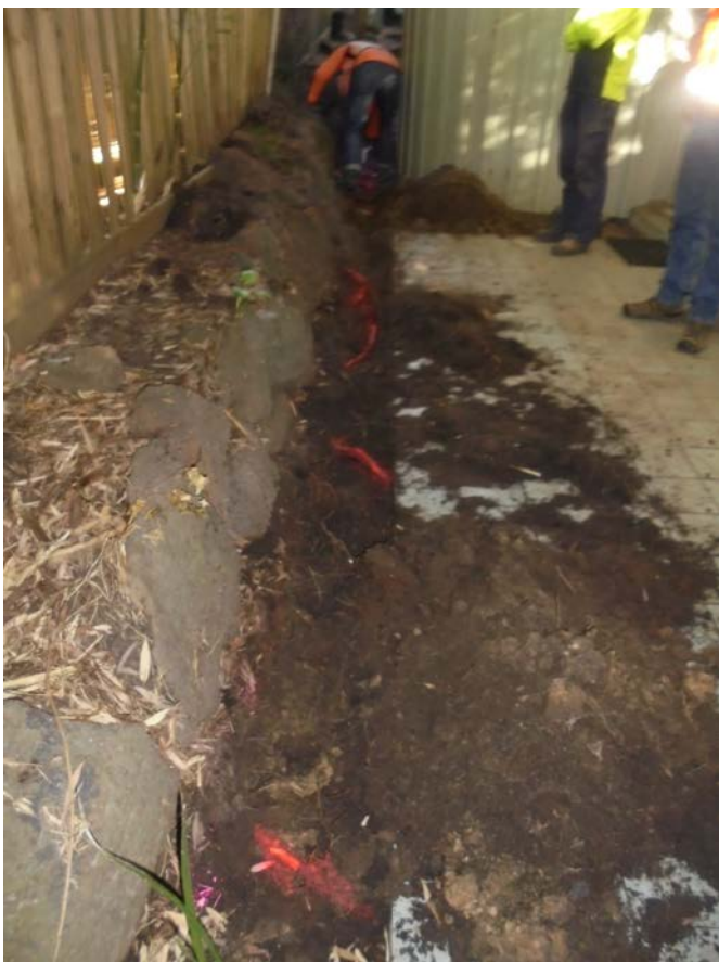
Figure 1: Shows the trench alignment adjacent to the group of conifers located in the adjoining northern property at 35 – 37 Regent Street, Mount Waverley. Exposed roots are highlighted in pink.
