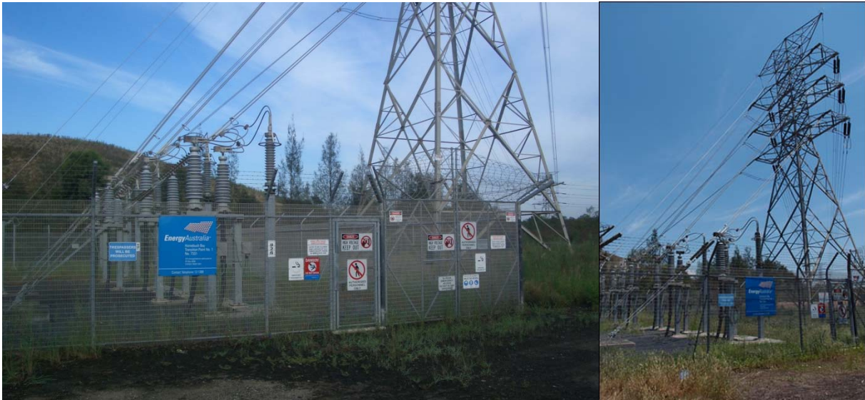
Figure 1 Guyed termination transition (Energy Australia, NSW)
