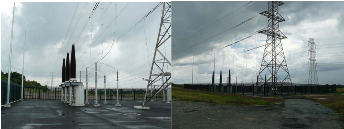
Figure 2 Extended insulation dropping arrangement (Powerlink, QLD)
