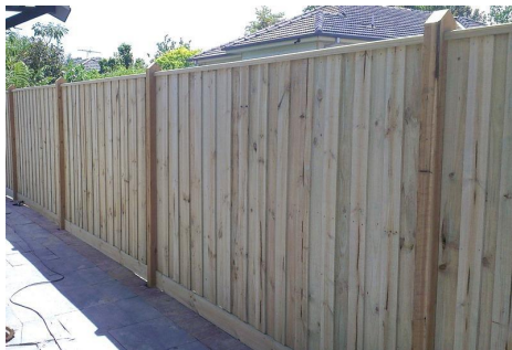
ACOUSTIC AND BOUNDARY FENCE
